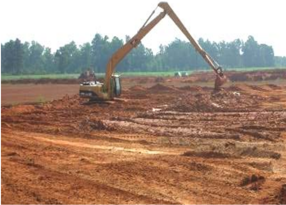
Figure 13. Area of high slimes content being excavated and mixed by “dipping”. This process helps to homogenize the final reclamation surface with respect to soil texture. Photo courtesy of Chuck Stilson/Iluka.
