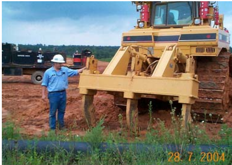
Figure 21. Deep shank ripper used to cross-rip experimental plots at Old Hickory. This ripping practice is now utilized for all newly reclaimed lands at Old Hickory.
