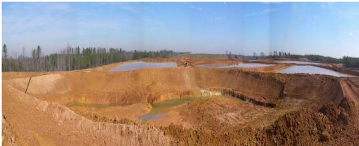
Figure 10. Mined out pit with dike walls ready to receive tailings return. The pits in the background are in the process of settling and water decant. The topsoil berms are outside and away from the inner dike walls. Photo courtesy of Chuck Stilson/Iluka.
