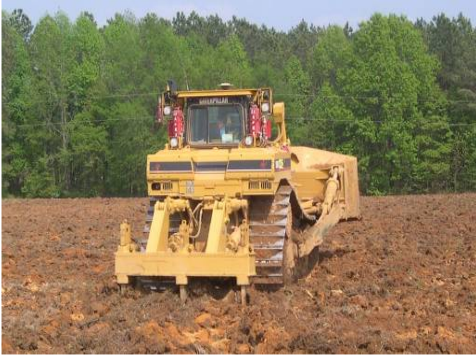
Figure 14. Three-shank ripper being used to rip topsoil and subsoil in one pass. The ripper shanks are pulled to approximately 75 cm. For our experiment on the Carraway-Winn Reclamation Research Farm, the subsoil was ripped in two directions (90°) after the lime and P were applied. The topsoil was then returned over the ripped subsoil and loosened again with a chisel plow. Photo courtesy of Chuck Stilson/Iluka.
