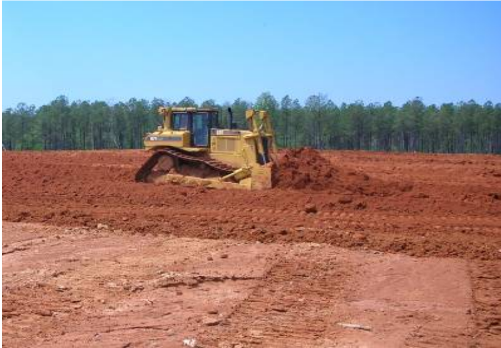
Figure 2. Final grading of mixed tailings and slimes at Old Hickory. Lime and P are added to this surface and mixed with chisel plow before the topsoil is returned. Photo courtesy of Chuck Stilson/Iluka.
