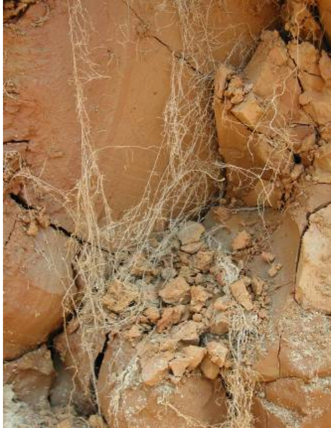
Figure 37. Root masses along desiccation cracks exposed after soil pit was excavated. This was high slimes C horizon material that had obviously dewatered and consolidated over time, leading to the development of large polygonal structural units.
