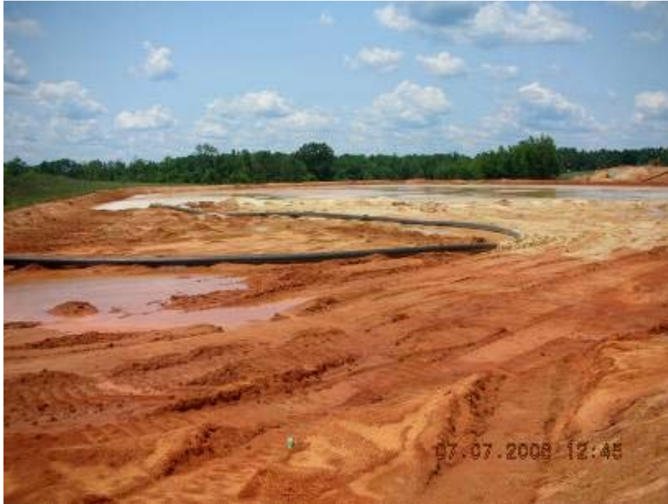
Figure 12. Backfilled pit receiving final capping of sandy tailings. Photo courtesy of Chuck Stilson/Iluka.
