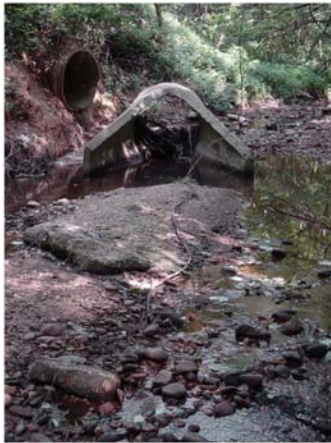
Figure 5: Undercut pipe discharge.
