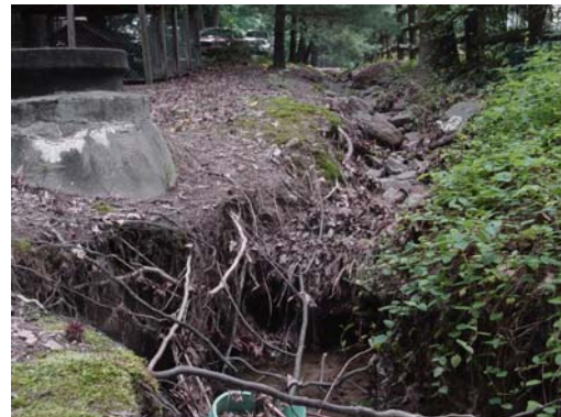
Figure 6: Undercut earthen and rocked discharge channel.
