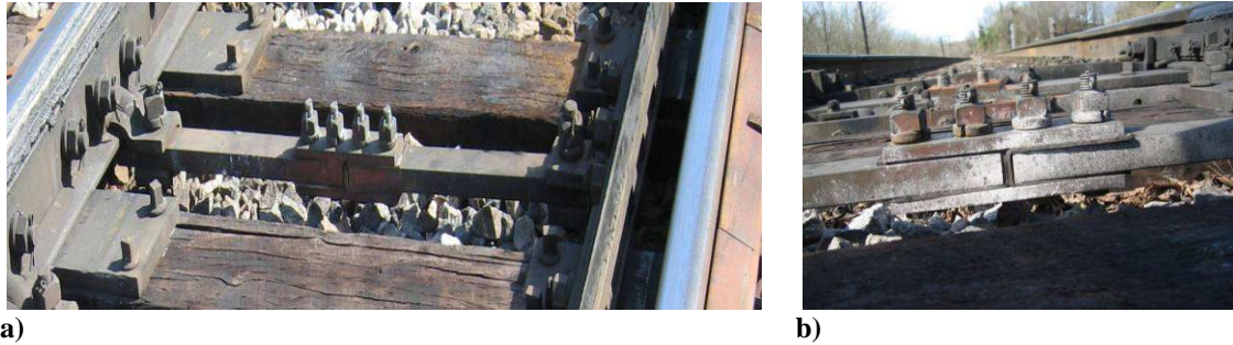
Figure 3.2. Snapshots of a) a switch rod and b) an insulated bolted joint
