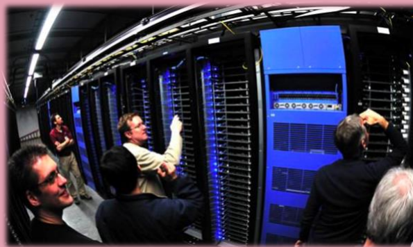
Figure 2. Facebook data storage center
