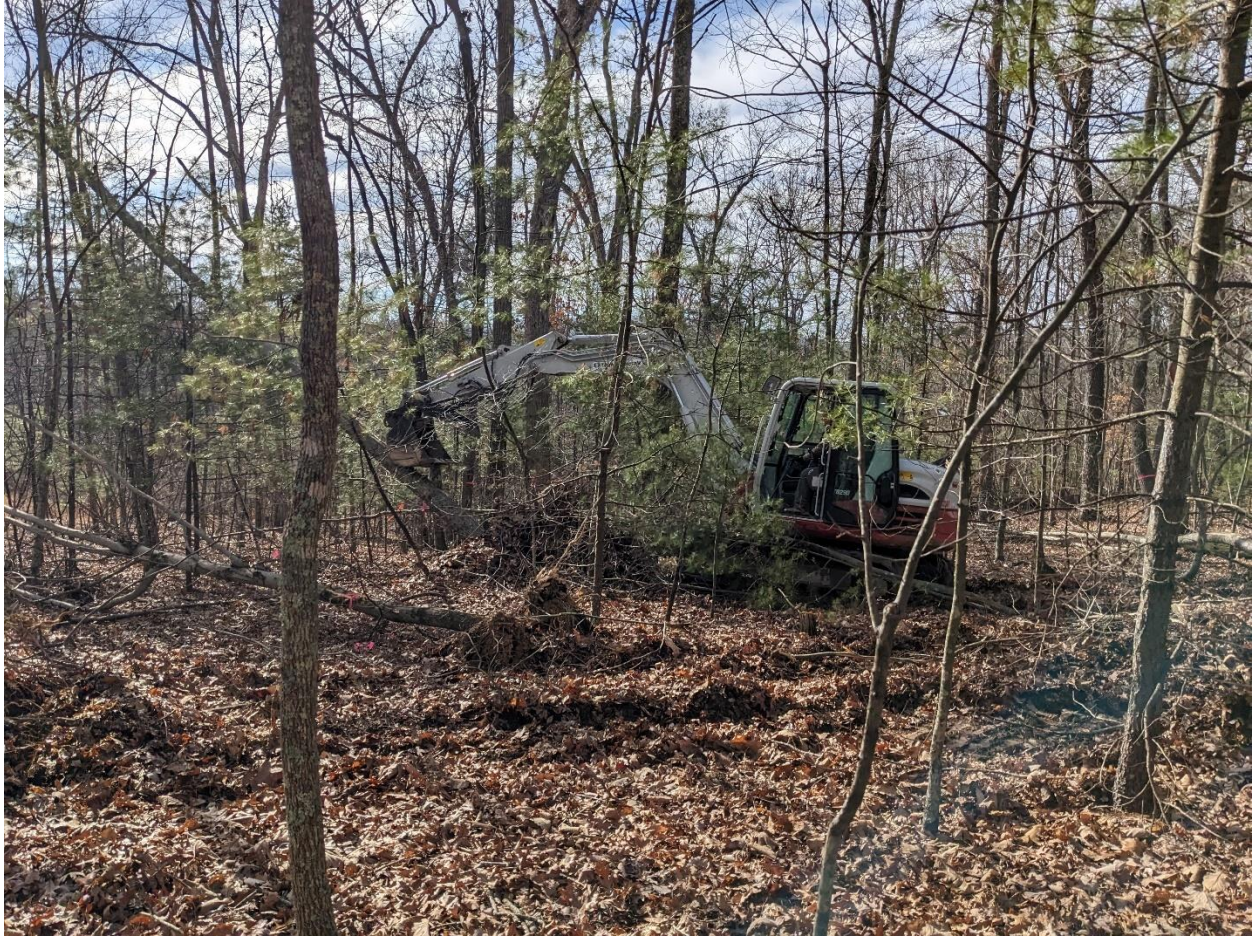
Figure 2.3. I used a Takeuchi TB290 compact excavator crane arm to push over eight trees (a density of 160 trees per ha) in each tip-up mound treatment unit for artificial tip-up mound creation in Virginia Tech's Fishburn Forest, Montgomery County, Virginia, USA.
