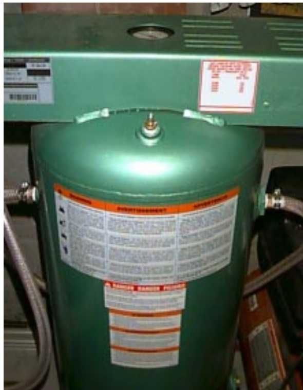
Figure 3.5. Constant Pressure Air Reservoir
