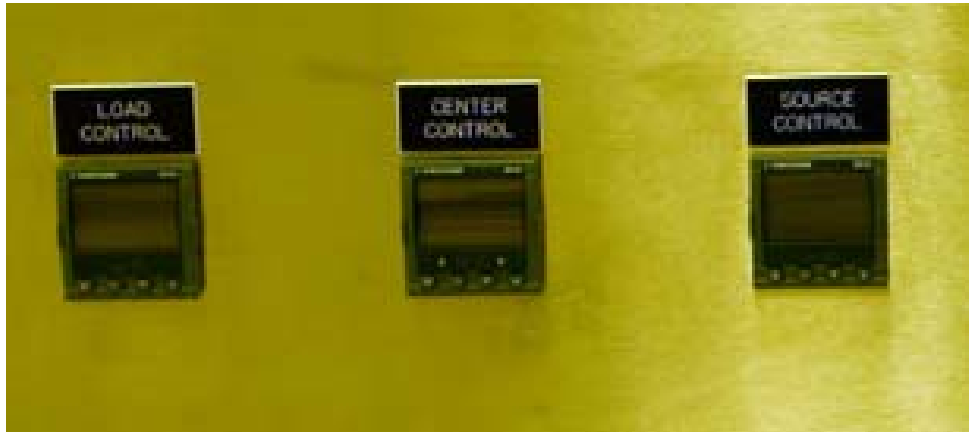
Figure 27 Enlargement of temperature controls. Center controller is set to desired temperature and other controllers are used to monitor the temperature at the front and back of the furnace.
