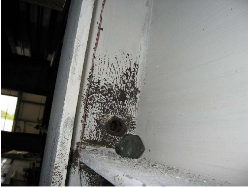
FIGURE 3.14: FAILED CONNECTION / INTERIOR BOLT RUPTURE, W27x84-SLAB
