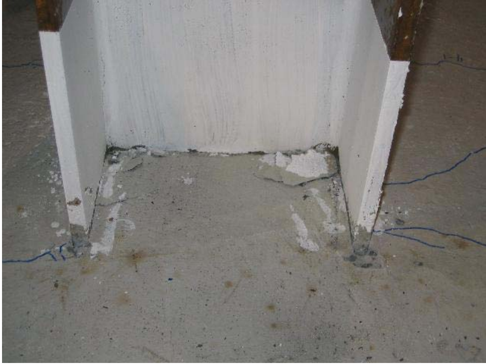
FIGURE 3.9: CONCRETE CRUSHING ON EAST SIDE OF COLUMN
