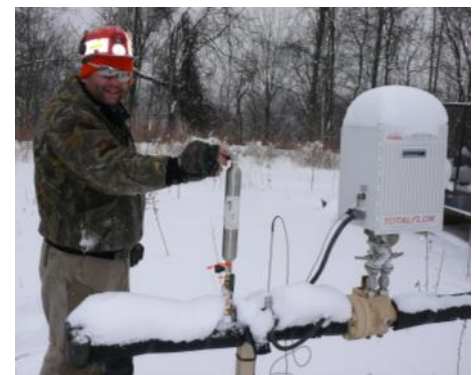
Dr. Ripepi working on the CO 2 injection project. As part of the study, one thousand tons of carbon dioxide were successfully injected into a coalbed methane well in Russell County, Virginia.
