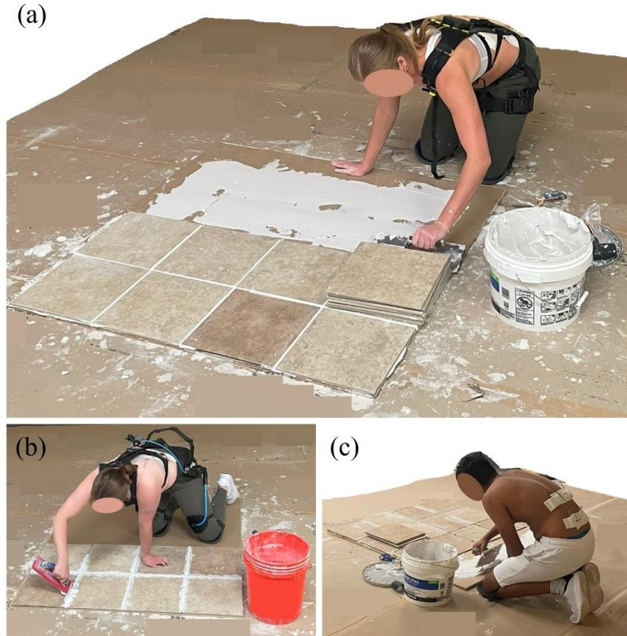
Figure 1. Illustrations of the tasks simulations: (a) tiling using the HeroWear Apex (HW); (b) grouting using the Laevo Flex (LV); and (c) tiling using No Device (ND).
