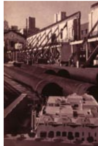
during renovation, brick walls stabilized (note model of new building in lower right corner) (40)
