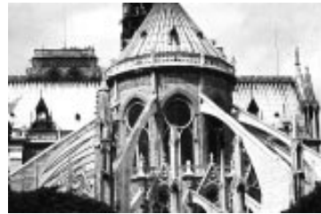
At Notre Dame Cathedral in Paris, France, flying buttresses elegantly resist the lateral forces of the roof.
