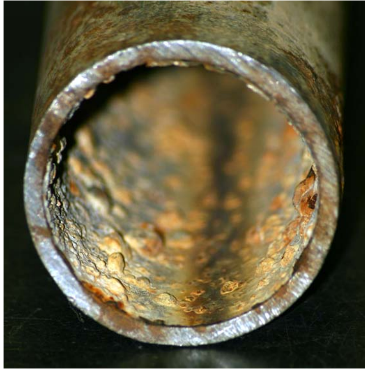
Figure 2-5. Corroded surface scales on the iron pipe (Photograph taken by Karen Blevins).
