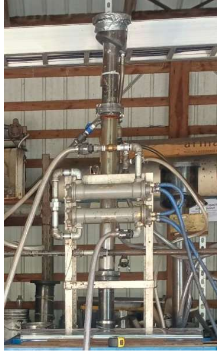
Figure 4.4: Phase separator upgrade.
