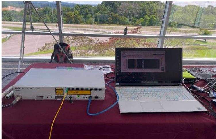
Figure 9. Photo. Fiber connection to NEC equipment in Virginia Smart Roads control room.
