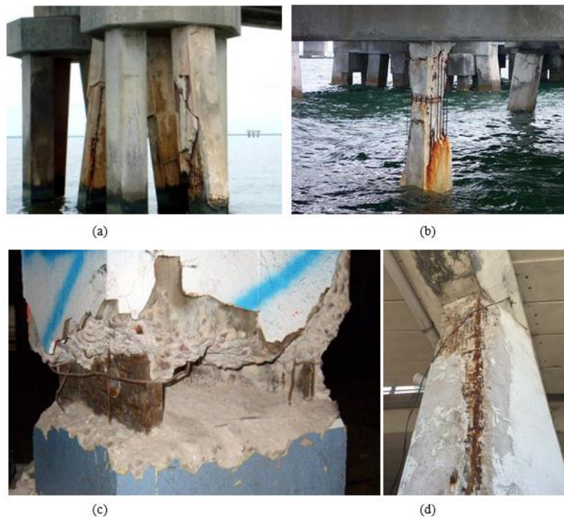
Figure 1.1: Concrete failures due to chloride-induced corrosion of steel in concrete, (a) corrosion of bridge pier and piles due to sea salt attack ((Moser et al, 2011), (b) bridge piling failure (NACE, 2014), (c) spalling of reinforced concrete pier (cpt, 2017), (d) delamination and spalling of the Gardiner Expressway's concrete in Toronto, Canada (Fahim, Giatech, 2018)
