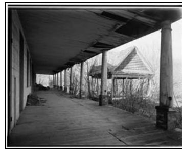
(Fig. 3.7) Sweet Chalybeate Springs, Spring House (Library of Congress), Prints and Photographs Division FROM PORCH OF MAIN BUILDING HABS VA,3-SWECH,1E-1
