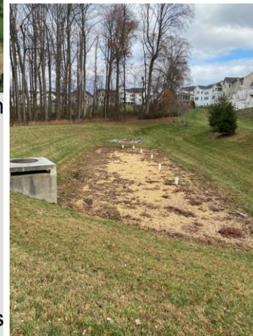
Sand Filter (SF) and inlet of Underground storage (UGS)
