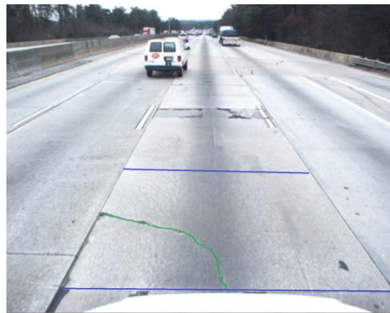
FIGURE 5 Pavement condition on I-285.
