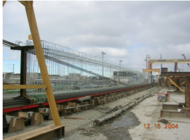
Figure 3. 4: Curing bed with steel layout, and steam distribution pipes located at base of bed.
