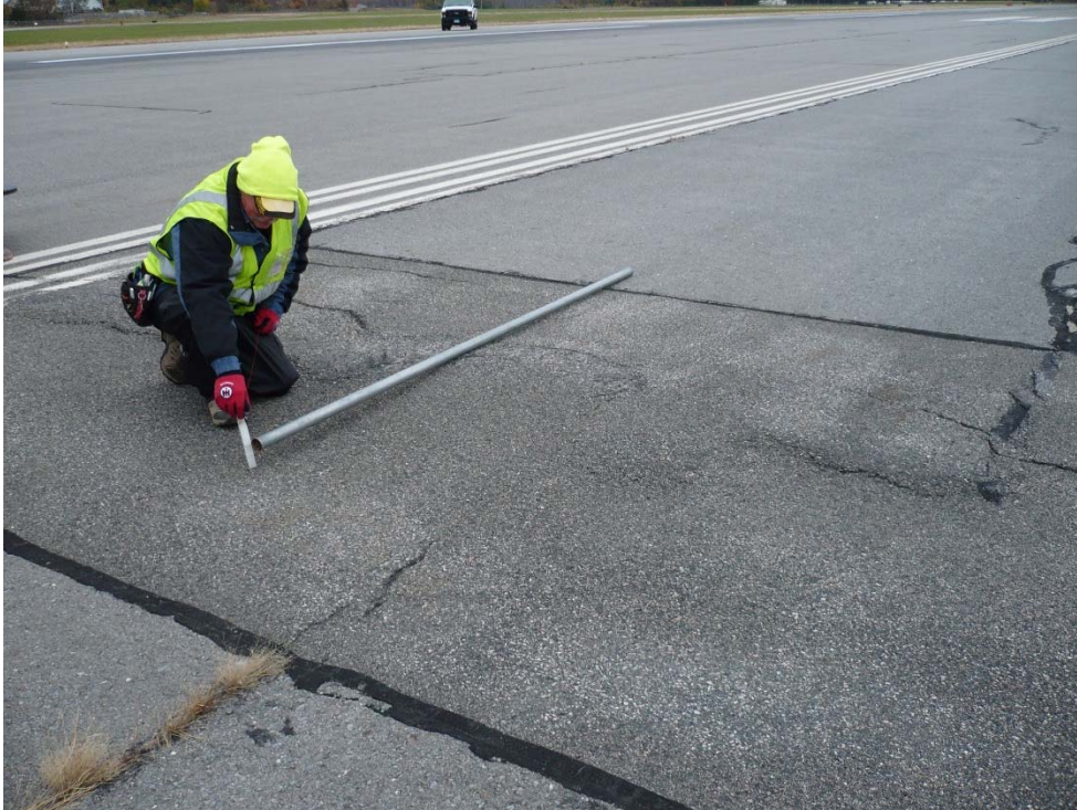
FIGURE 1 Measurement of Pavement Depression with 10-Foot Straight Edge.
