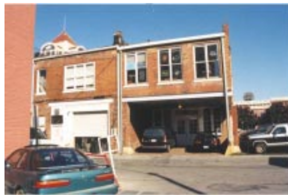
Condition of artist's studio facing parking lot (15)
