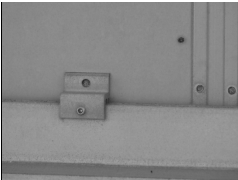
Figure 11. Failed Stud on Sign.
