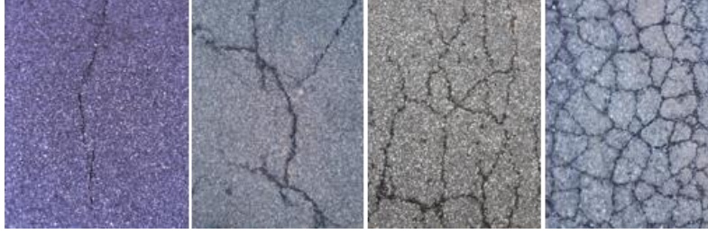
Figure 2.18. From left to right: LT, LA, MA, and SA cracking networks.
