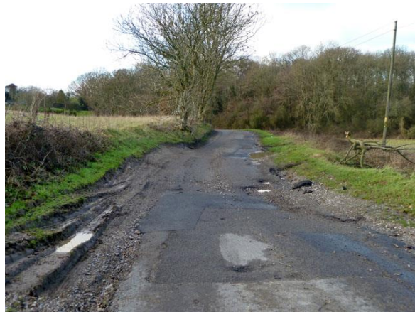
Figure 1.1: Road in disrepair. Public Domain.
