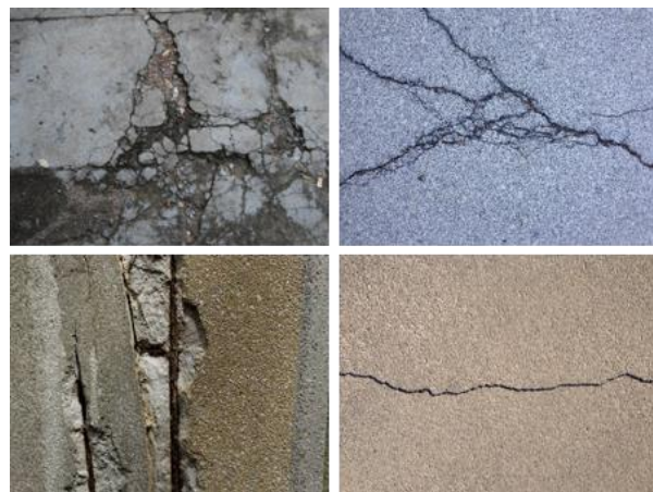
Figure 1.2: Concrete distress. From top left to bottom right: punch-out, cluster cracks, spalling, and longitudinal/transverse crack. Public Domain.
