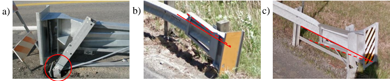
Figure 4-3 Severely damaged ET-Plus: a) S1; b) S2; c) S3
