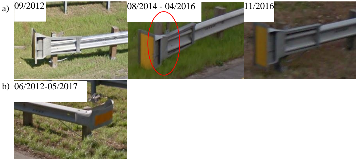
Figure 4-6 Examples of damaged end terminals in use along U.S. roads: a) an ET-Plus end terminal that was damaged during 2012-2016; b) a BCT end terminal which was damaged since 2012
