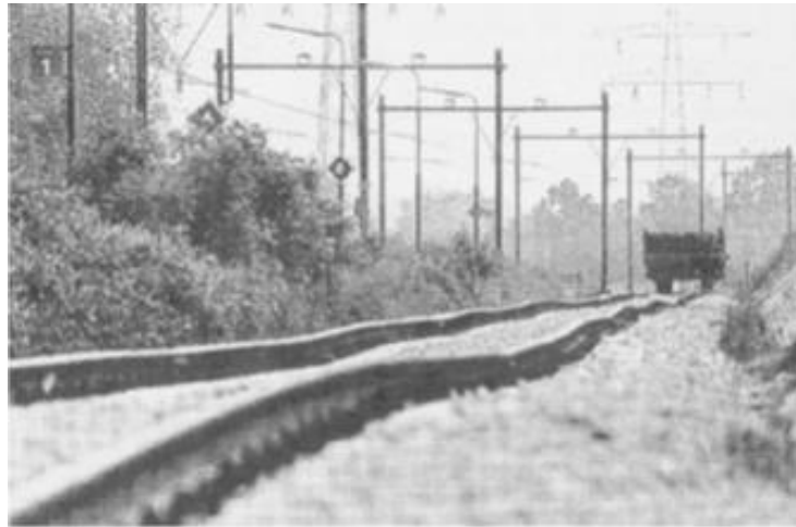
Figure 2.2 Defects in railway track geometry caused by settlement of ballast, image sourced from [9].
