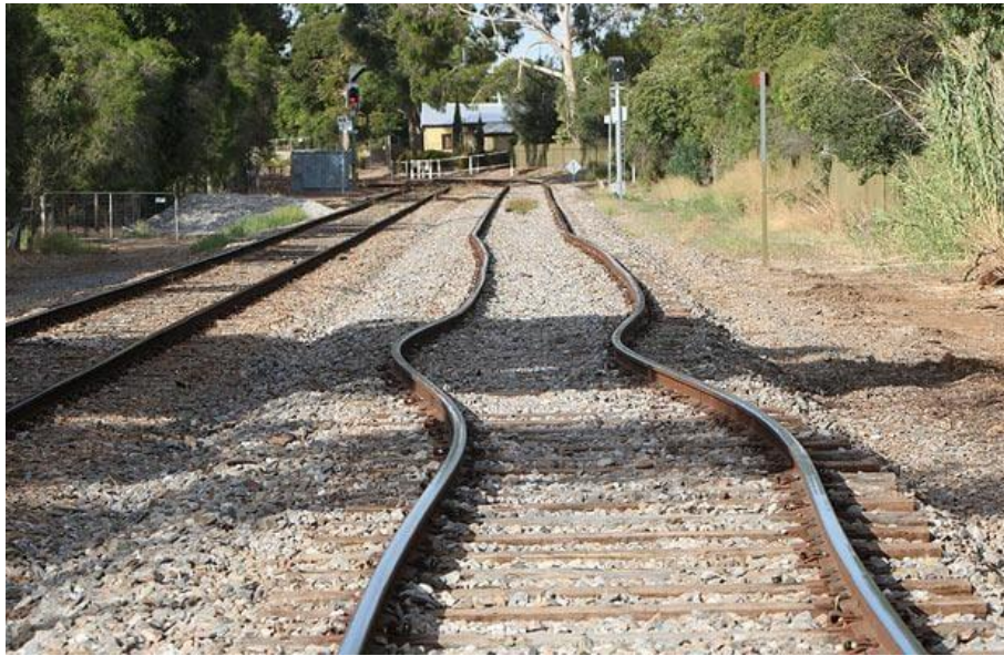
Figure 2.3 Buckling of railway tracks in the lateral direction due to thermal stresses [10].
