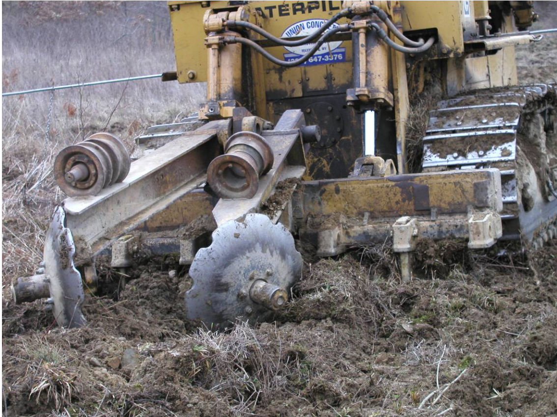
Photo 1. An advanced ripping tool used to prepare the biomass research sites by Union Concrete Products of Maxwellton, West Virginia, under the direction of J. K. Rose.
