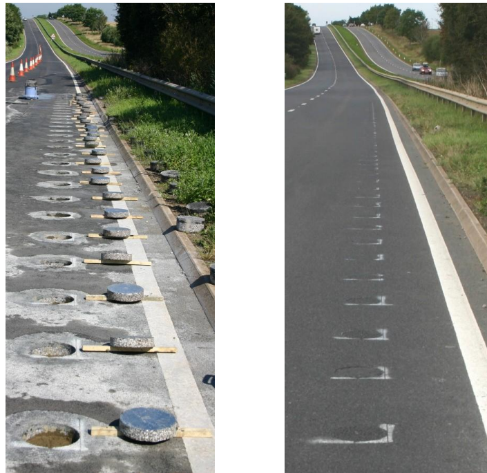
Figure 2 - Asphalt discs in site C about to be installed (left) and shortly after installation (right)
