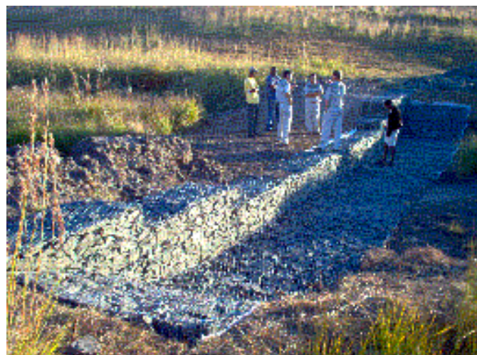
Gabion structures in the Oribi loop within the Golden Gate National Park
