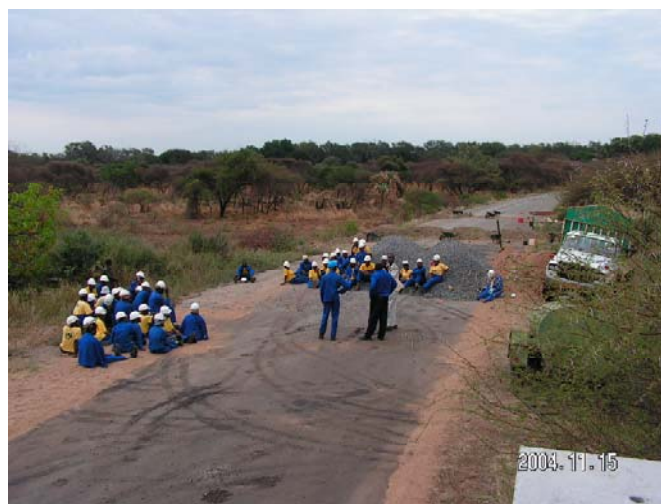
Inserting 11 sets of culverts across tourist route in the Kruger National Park to enhance water flow in Luvuvhu river flood-plain
