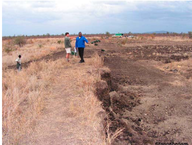
More than 8000 m 3 of dam wall are removed and transported to old gravel pits. Stangene dam, Kruger National Park
