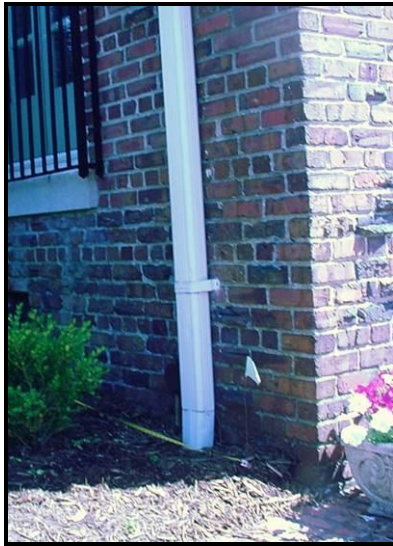
Figure 5.13 Residence A front downspout directed belowground Adrienne J.L. Tucker
