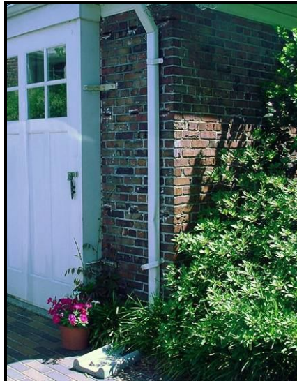
Figure 5.14 Residence A garage/in-law apartment downspout directed onto the driveway Adrienne J.L. Tucker
