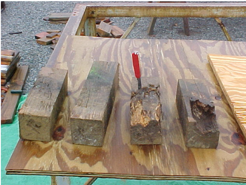
Figure 2- 15. Decayed portion of 4x4 posts of Deck No. 6 that were in ground contact while in-service.
