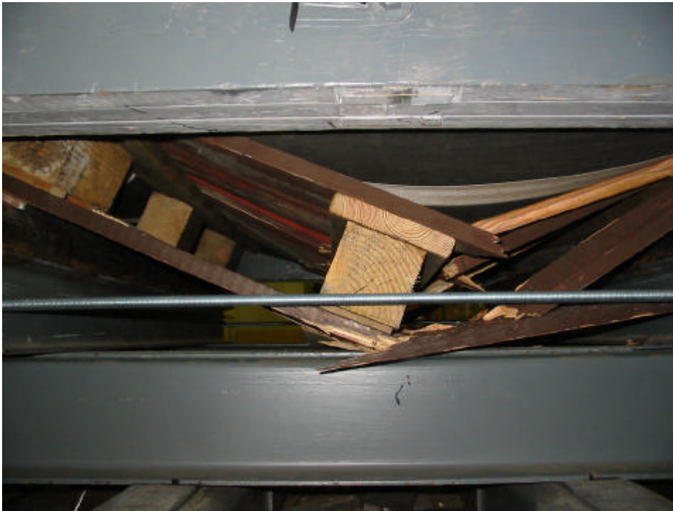
Figure 4- 16. Block pallet racked across the width after failure.
