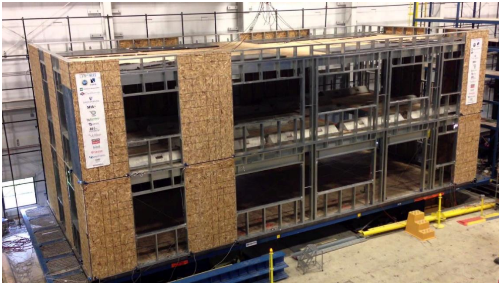
Fig. 2.1. Full-scale CFS framed building seismic test. Peterman, K., Stehman, M., Buonopane, S., Nakata, N., Madsen, R., and Schafer, B. (2014). "SEISMIC PERFORMANCE OF FULL-SCALE COLD-FORMED STEEL BUILDINGS.", Tenth U.S. National Conference on Earthquake Engineering, Anchorage, Alaska. Used under fair use, 2015.
