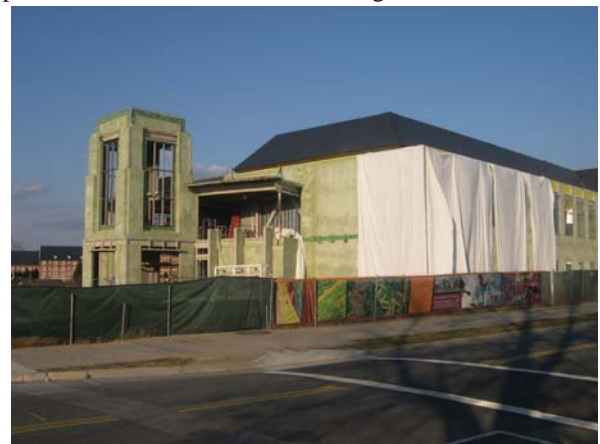
Construction is proceeding rapidly for Life Science I building on Washington Street (photo taken December 2006)
