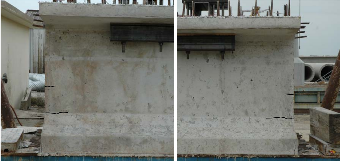
Figure 37. Crack Pattern in the 12 ksi Anchorage Zone After Lifting
