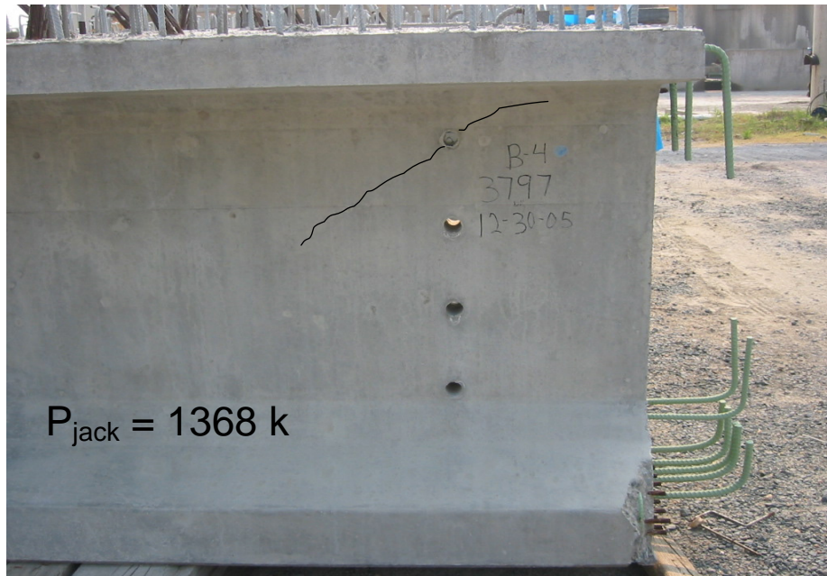
Figure 16. PCBT-53 Anchorage Zone Case Study – Fair Condition
