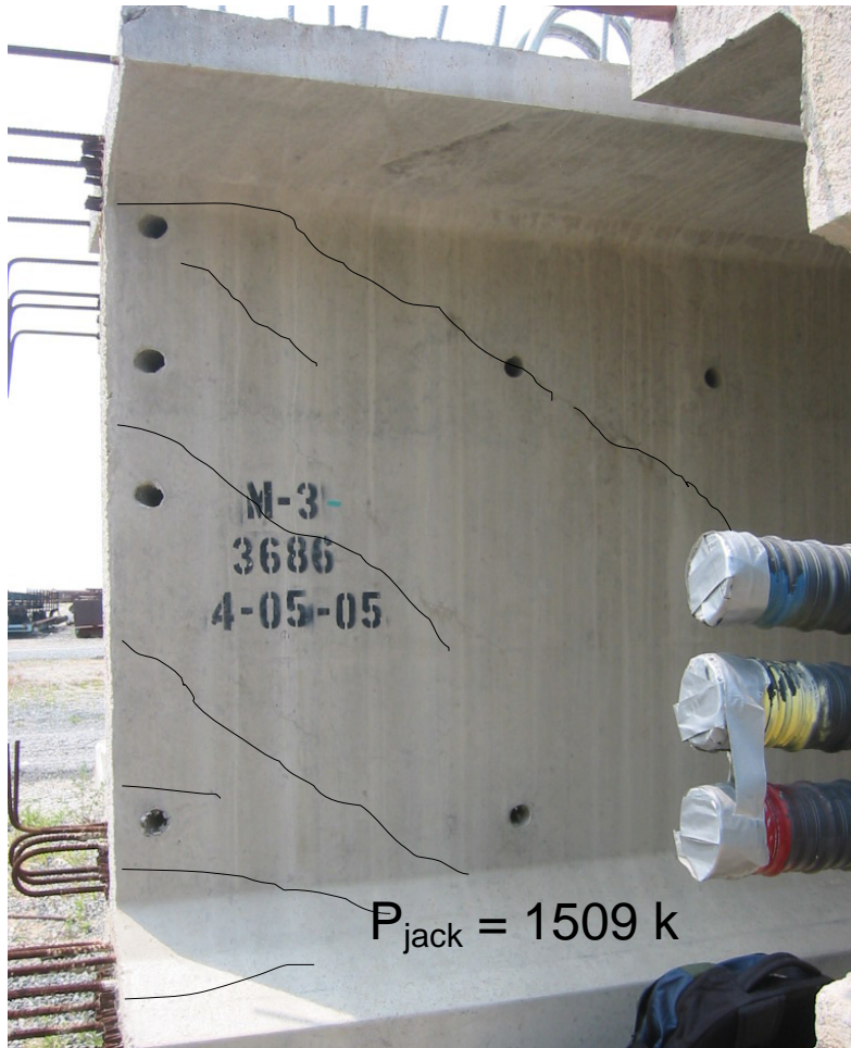
Figure 18. PCBT-77 Anchorage Zone Case Study – Poor Condition
