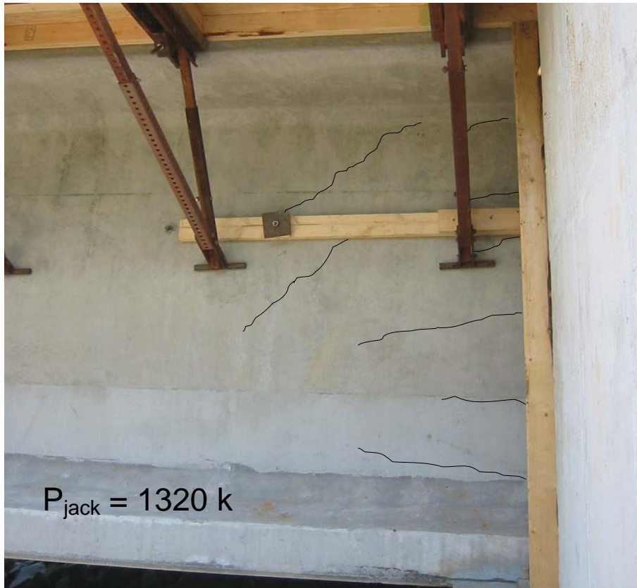
Figure 19. PCBT-77 Anchorage Zone – Poor Condition
