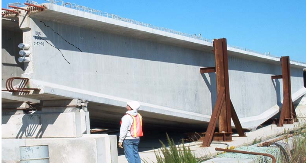
Figure 22. Anchorage Zone Cracking Observed in Deep Haunched Girders
