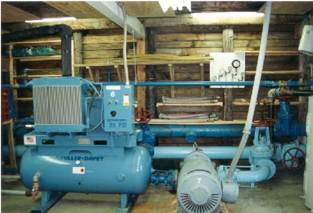
Figure 4.3 The Pump Room
