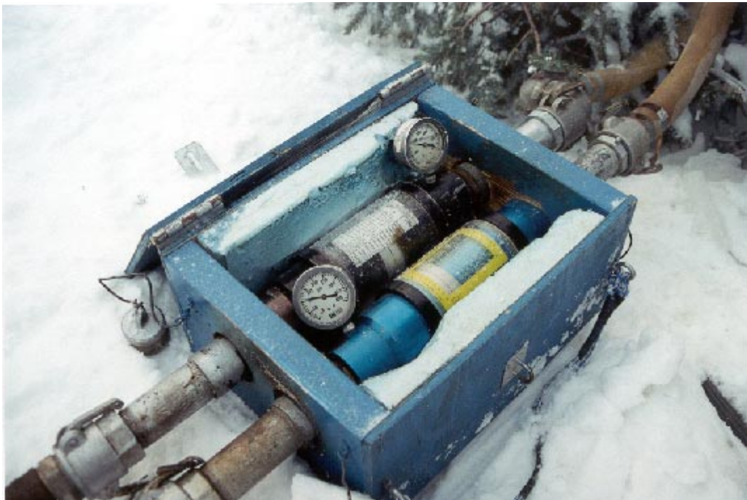
Figure 4.2 Air and Water Flowmeter
