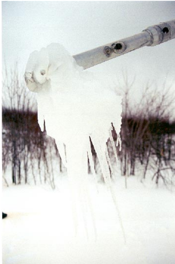
Figure 6.5 Frozen Tower Head and Nozzles
