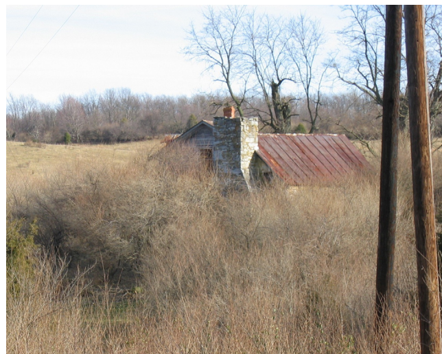
Autumn olive almost engulfing a structure
