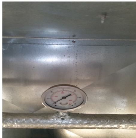
Figure A.1: Pressure readout in the chiller unit. Can be found by removing the diamond shaped panel on the outdoor chiller unit.
