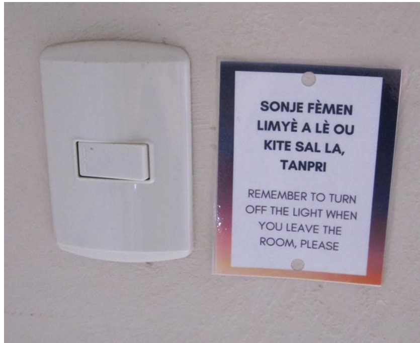
Figure 3.1: The light switch tags that a JustEnergy board member posted in the Haitian hospital that the group was installing a solar panel array
