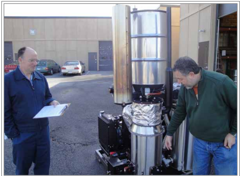
Rick Caudill, SBIO Department’s Technician, takes notes from biomass international consultant Yaov Palatnik during the generator’s commissioning process.
